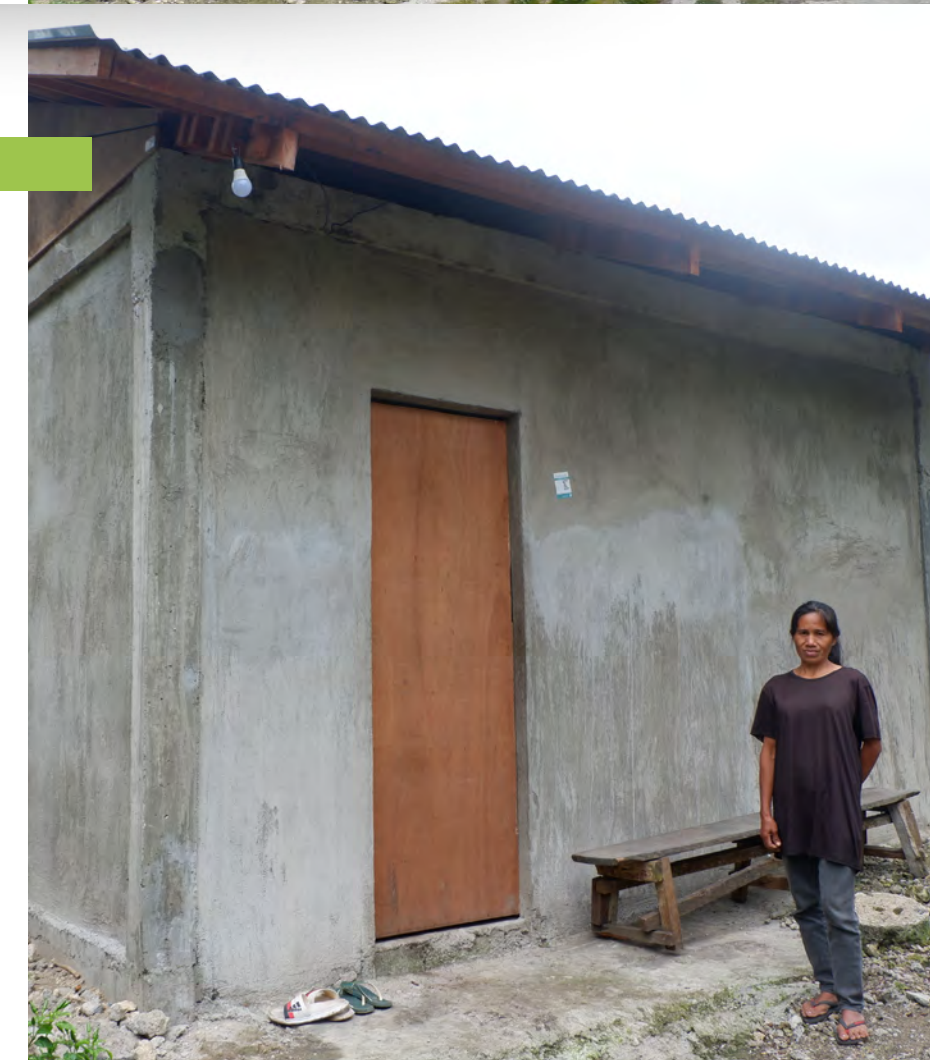
Build Change and microfinance partner ASA Philippines supported Deoclesa (right) and Carmela (above) to retrofit their homes in Carcar City, Cebu.
